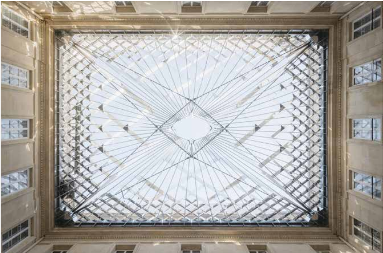
The glass roof designed by Hugh Dutton © Nicolas Trouillard – Centre des monuments nationaux.
